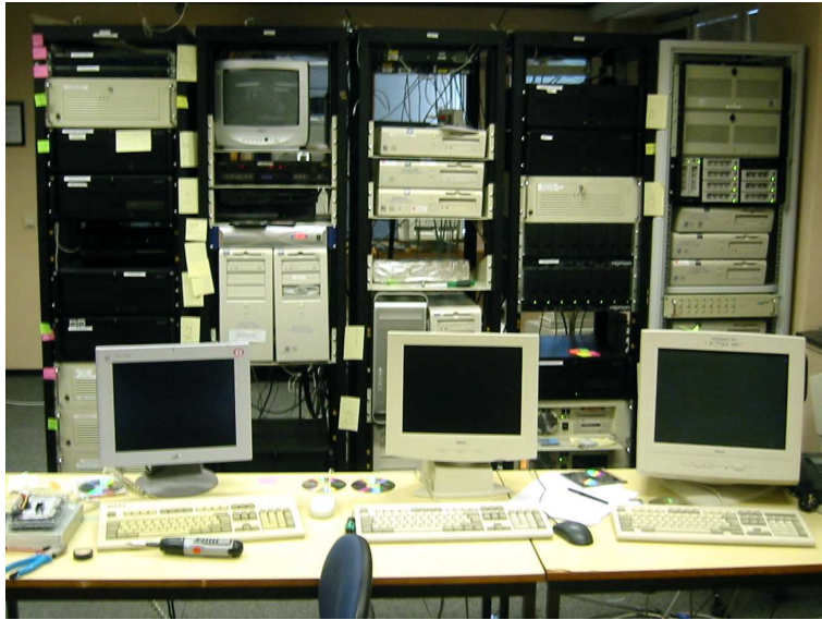
Figure G.10: Server room
